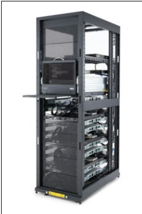
Figure 7. Rear View of System with Cabling
